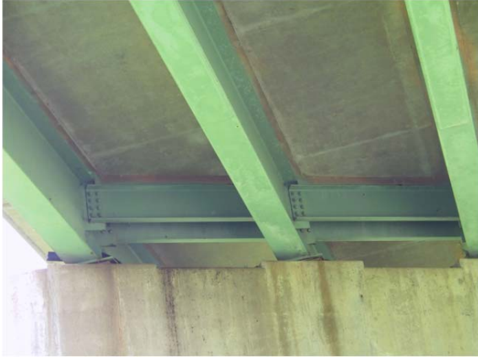
Photo 10: Guano staining on side of pier
