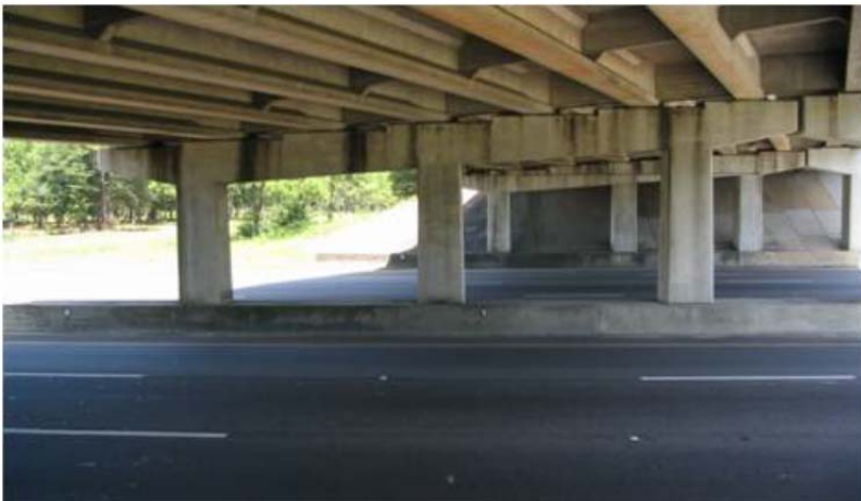
Photo 9: Staining on sides of pier caps
