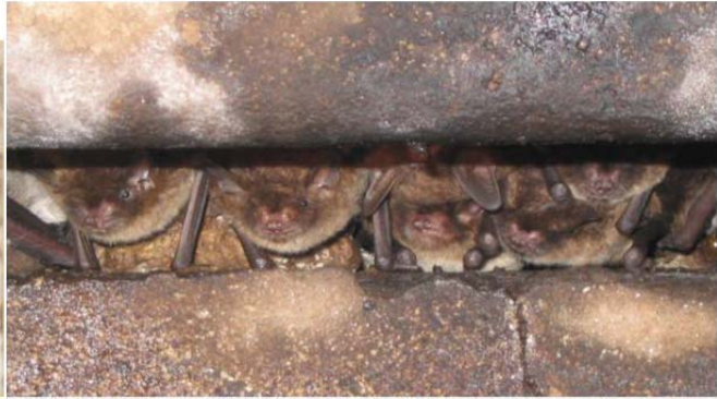
Photo 2: Visible bats within an expansion joint
