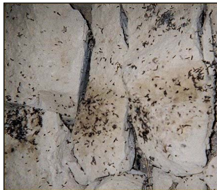
Photo 6: Bat Guano on Riprap
