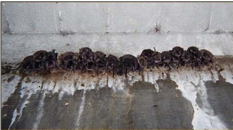
Photo 11: Bats Roosting & Associated Staining
