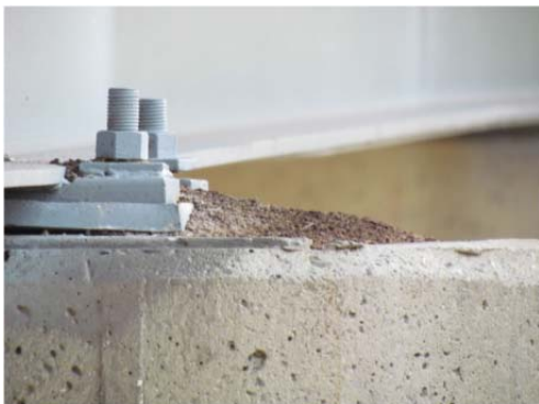
Photo 5: Guano deposit on pier, obscuring structural features.
